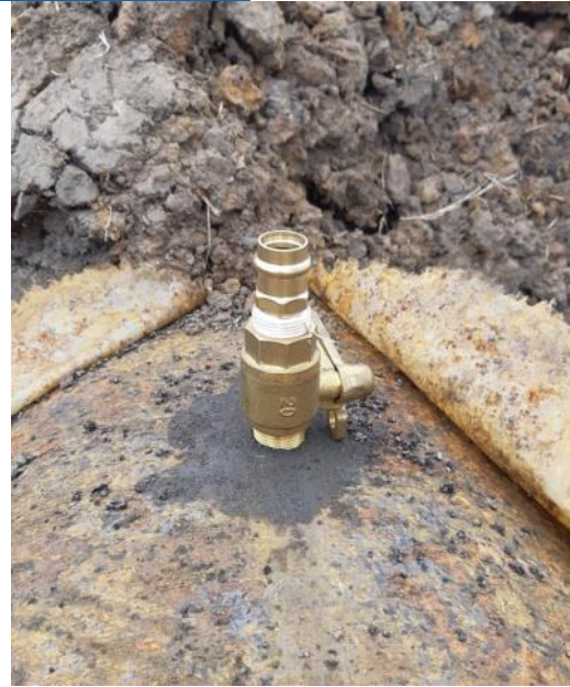
Figure 11. Monitoring pipe / Pressure release valve
