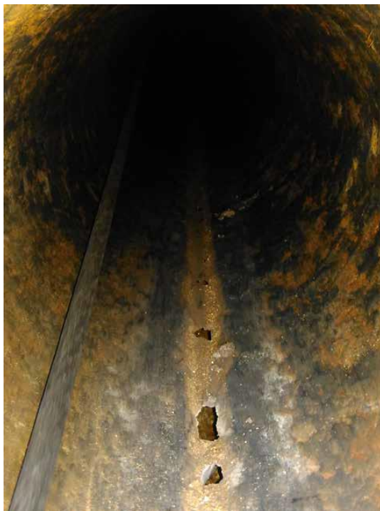
Figure 19. Pin holes in host pipe
